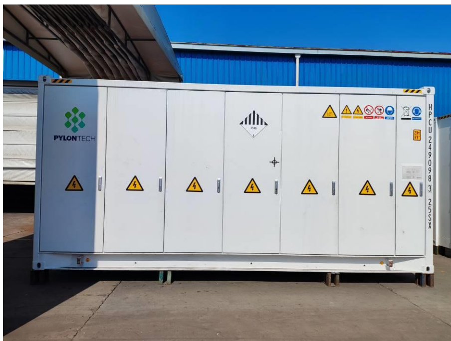
外观 (PowerCube-20H-M7A200C5.015-EU-05 电池系统) Appearance (PowerCube-20H-M7A200C5.015-EU-05 battery system)
